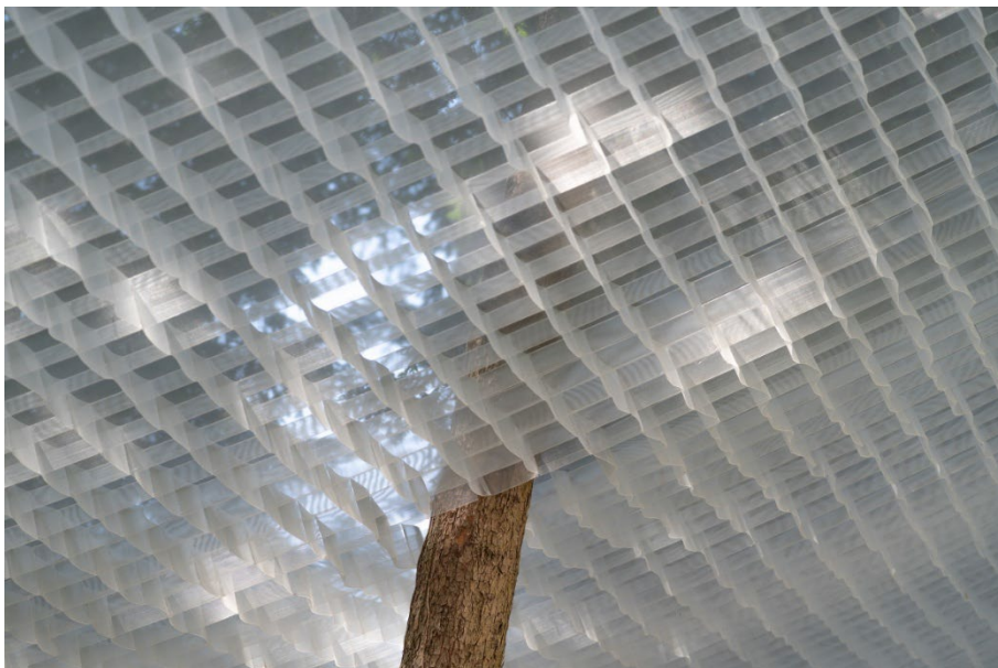
Figure 3. Textile Roof is made of a layer of three-dimensionally woven fabric. The layer consists of 100m 2 of cells with 100mm-wide recycled polyester sewn by hand. ©Sandro Sulaberidze
